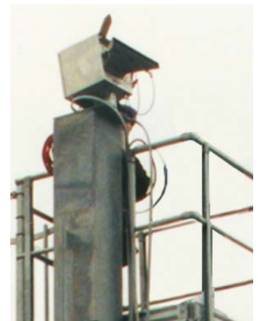
Linescanner in protective housing is mounted on top of a tower.
